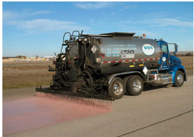
Asphalt pavement rejuvenator is applied to runway by Western Oil Spreading Services
